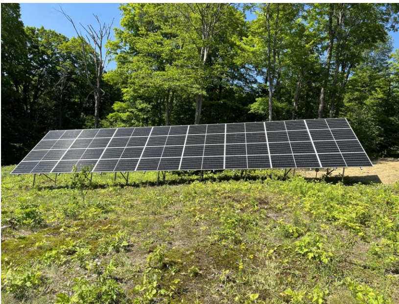
15kW residential solar array in Barnard
