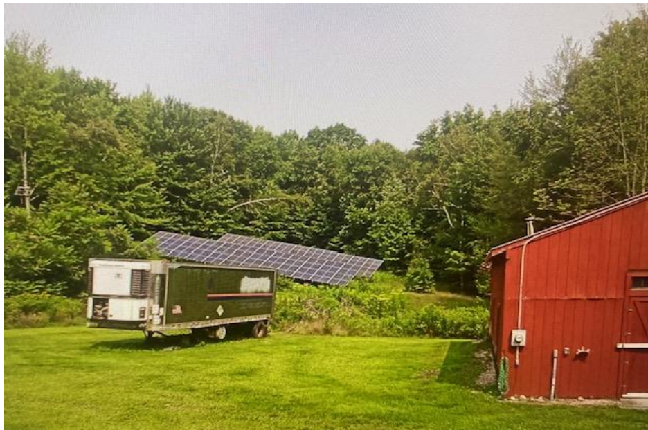
25kW residential solar array
